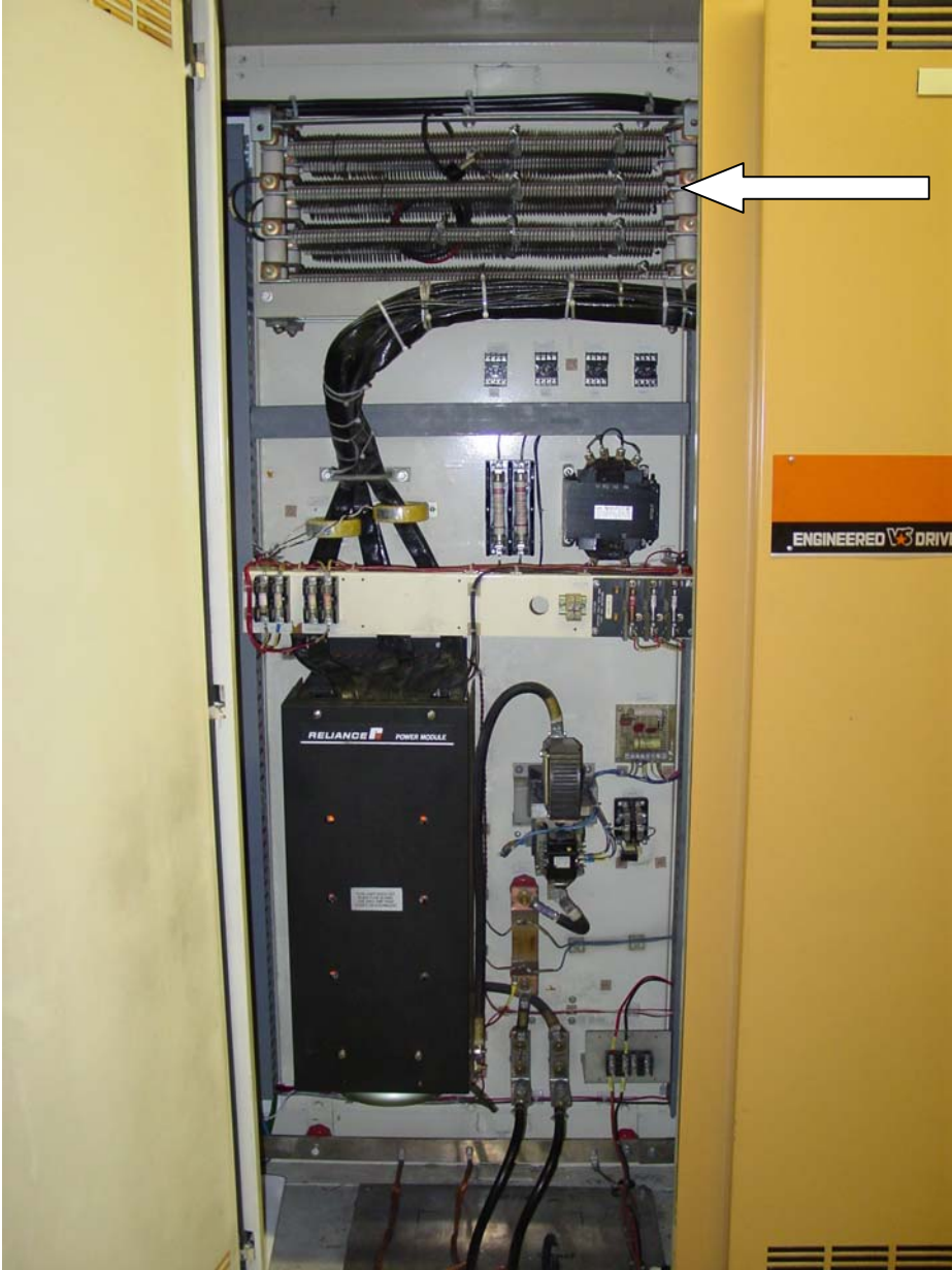
Obsolete reduced starting voltage resistor bank
