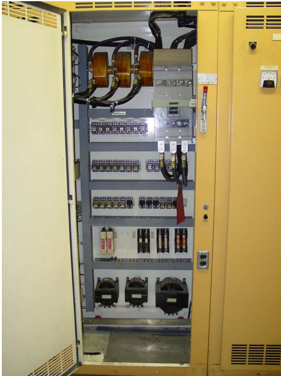
Domtar – Obsolete relays, fuses, and transformers.
