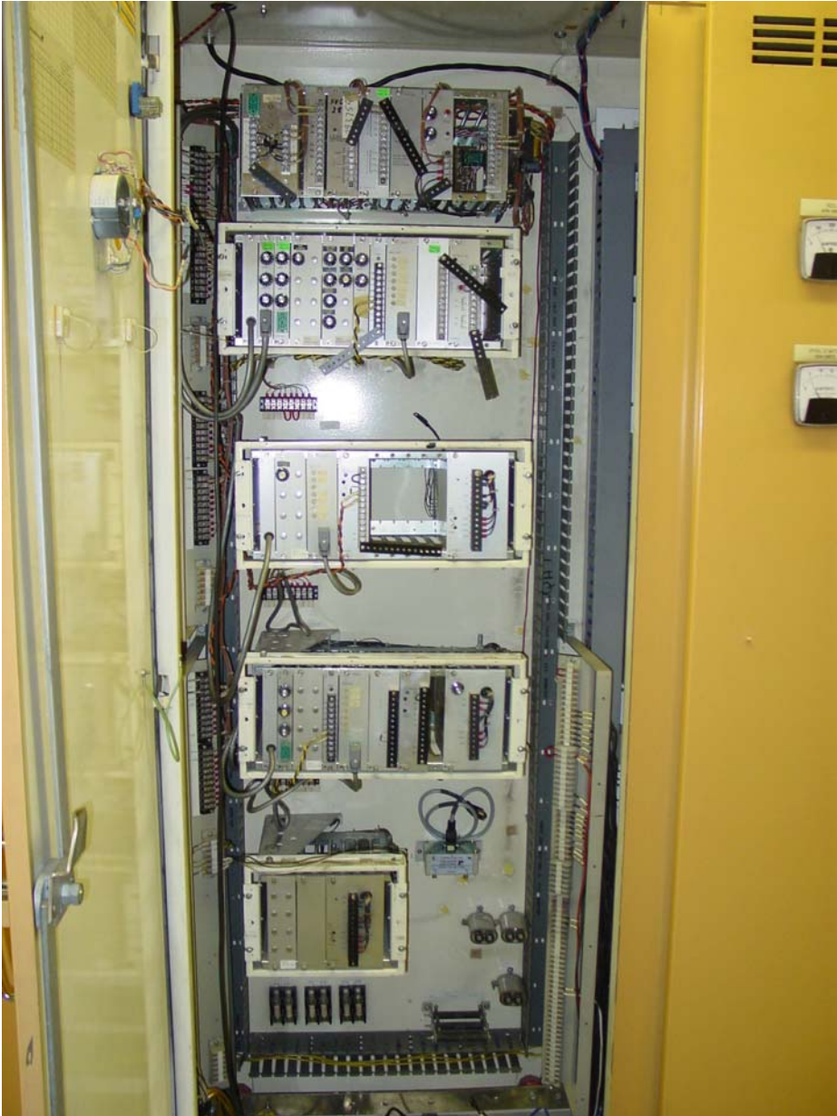
Domtar – Obsolete DC Drive
