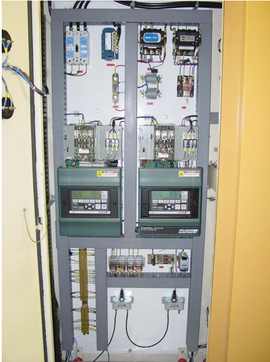
Domtar – Flexpak 3000 drives (Left: Standard Flexpak 3000 drive for Spool Starter.) (Right: Retrofitted Flexpak 3000 drive for Reel Drum.) (Top Right: Contactors for Field Reversing.)
